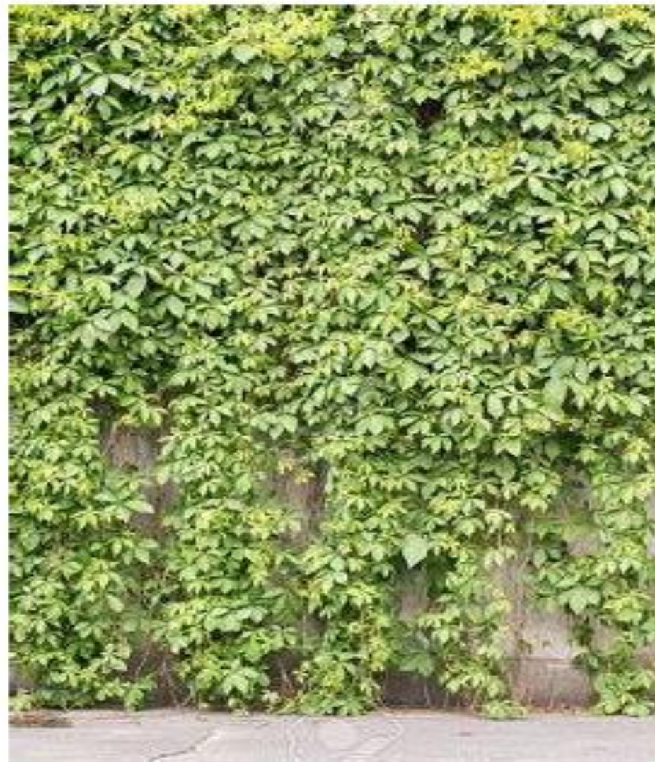
IVY CREEPER ON RETAINING WALL
